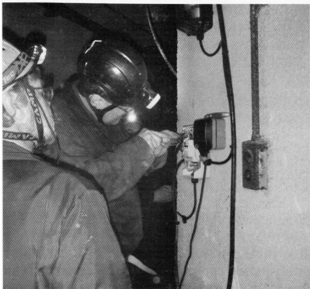
Dom and Mike and Bob connecting up new power and lights. Photo Ed Combes
